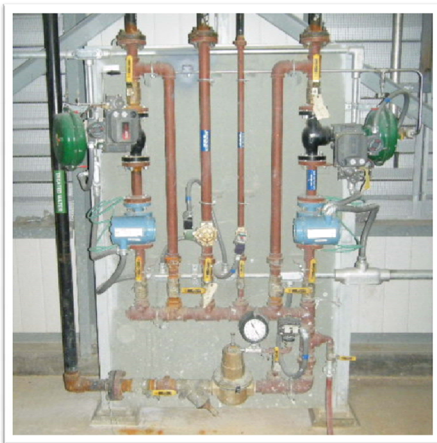
Water Control Panel
