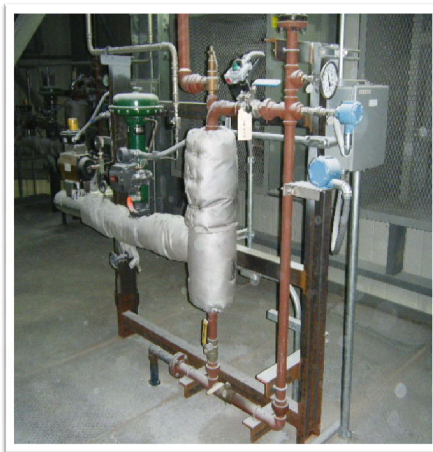
Slaking Water Heater
